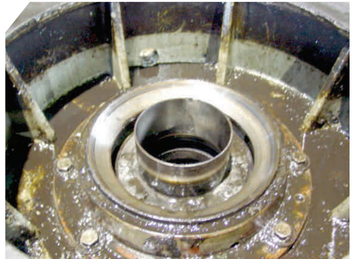
The damaged NDE bearing which was replaced before the motor failed.
